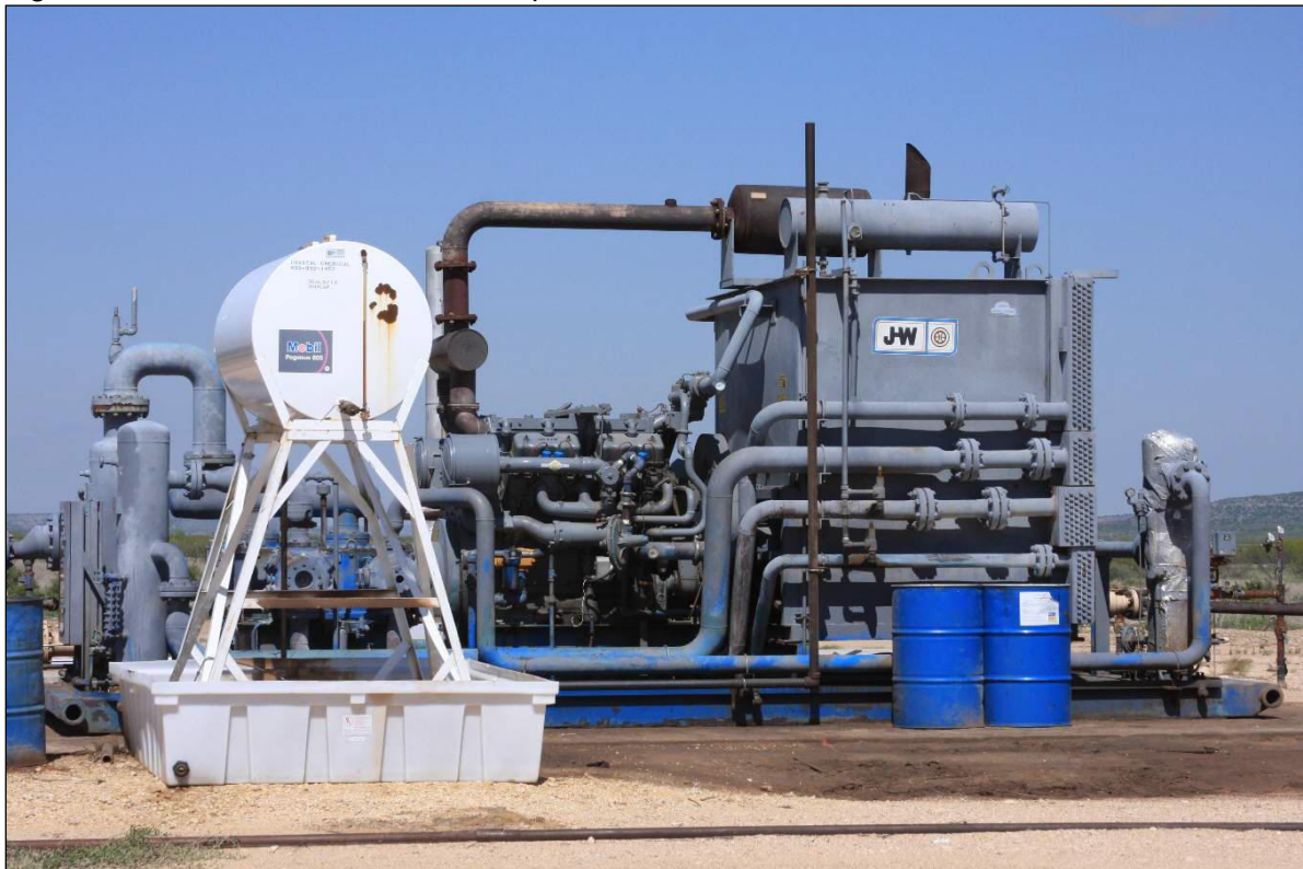
Figure 6-1: Photo of a Wellhead Compressor 297
