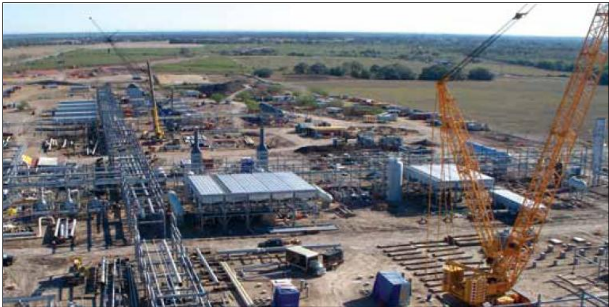
Figure 7-2: Processing Facility for Processing Gas Liquid under Construction in the Eagle Ford Shale
