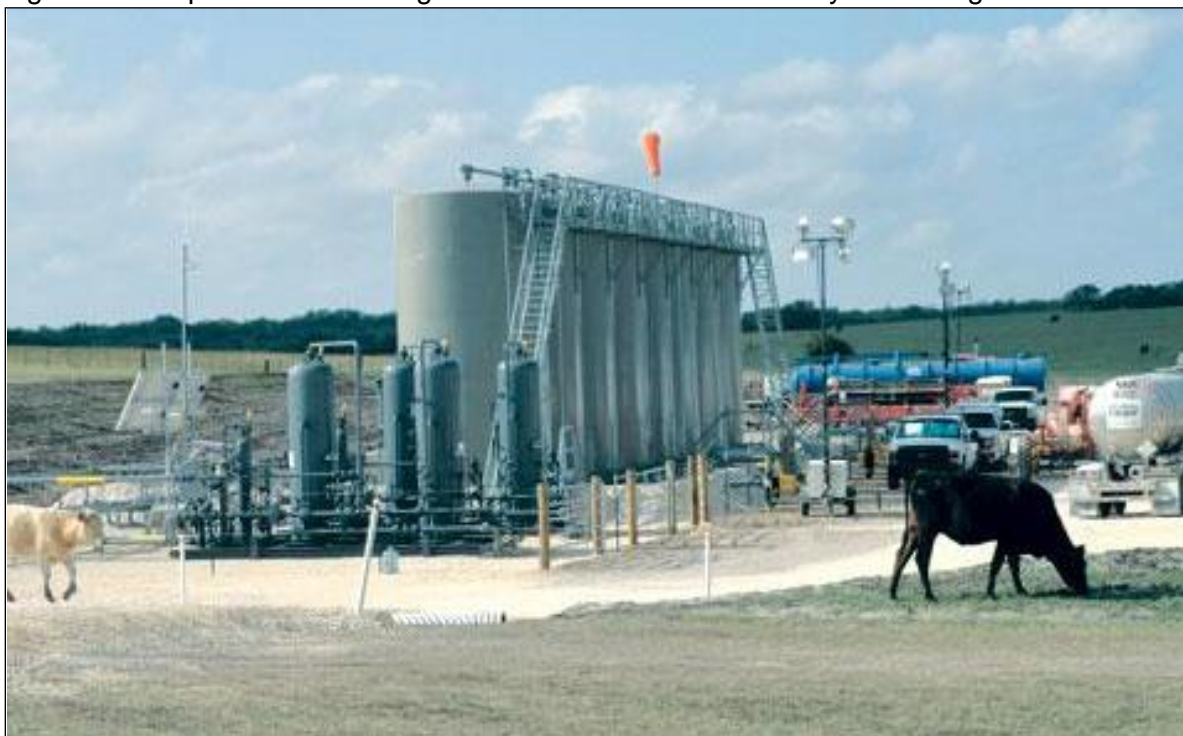
Figure 6-5: Separator and Storage Tanks at a Site near Kennedy in the Eagle Ford
