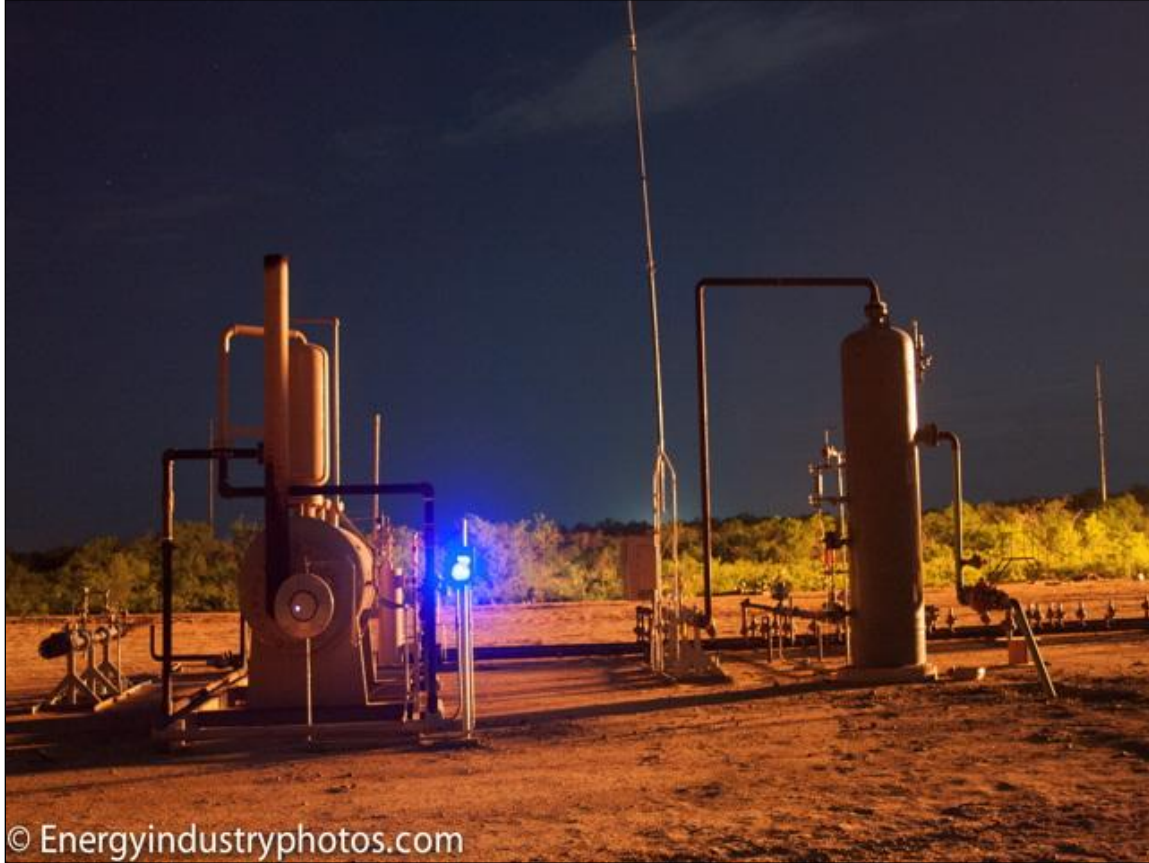
Figure 6-4: Dehydrator and Separator in Karnes County
