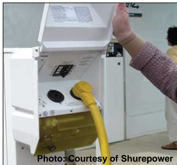
Figure 5-7: Shurepower Pedestal Hook Up
