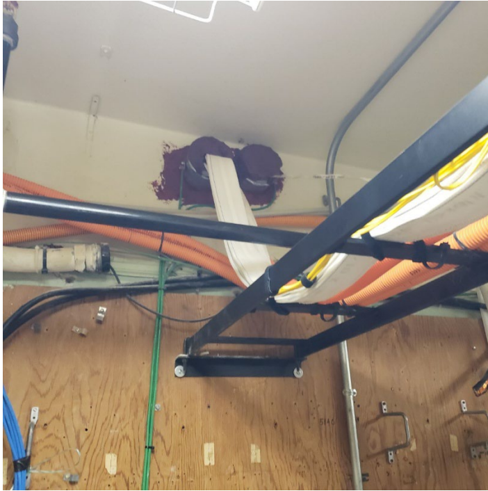
675 Comm Room Entrance Ducts
