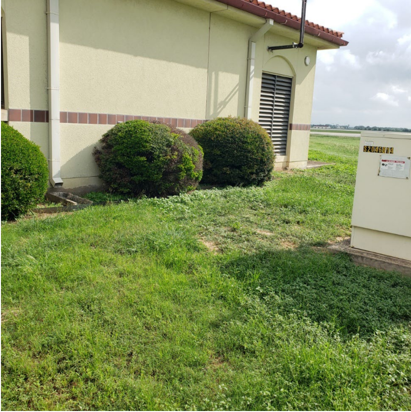
South Exterior Wall Generator Room
