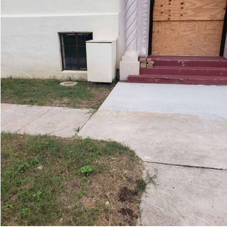
675 Exterior Pull Box
