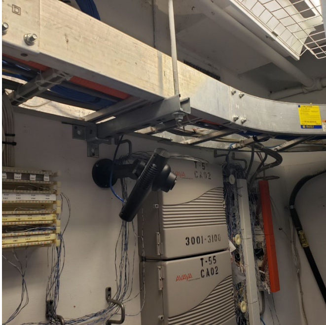
1 st Floor Equipment Room West Wall
