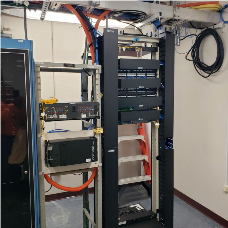
4 th Floor Equipment Room
