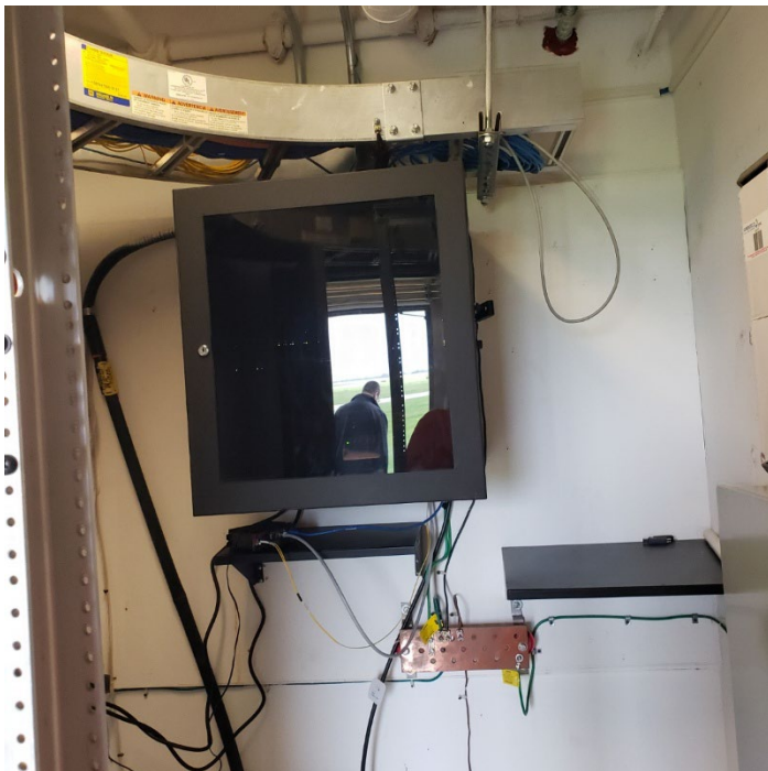
1 st Floor Equipment Room
