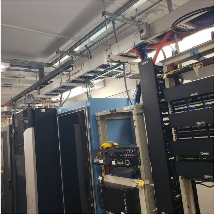
4 th Floor equipment room A
